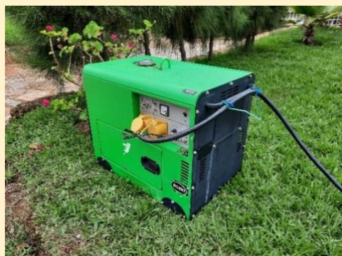
The generator and... ..
